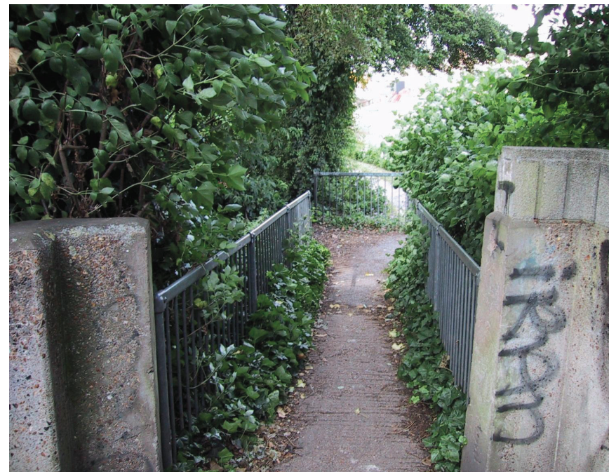
The Carlyon Road – Mount Pleasant pedestrian route was posed a perilous walk between a local school and deprived residential area with narrow, overgrown access ramps to the Grand Union Canal.
